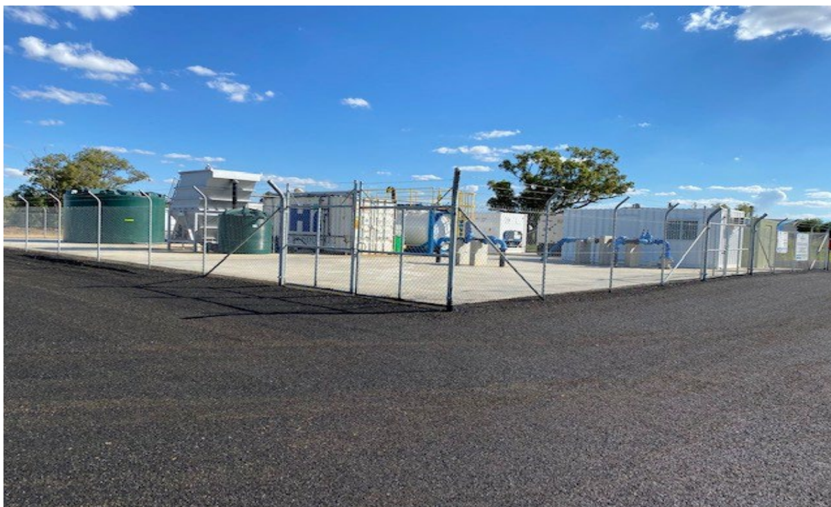
Narromine Temporary Drinking Water Treatment Plant
