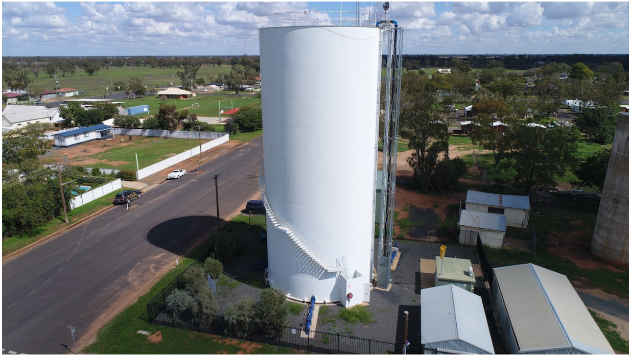
Trangie Drinking Water Reservoir and Chlorination System
